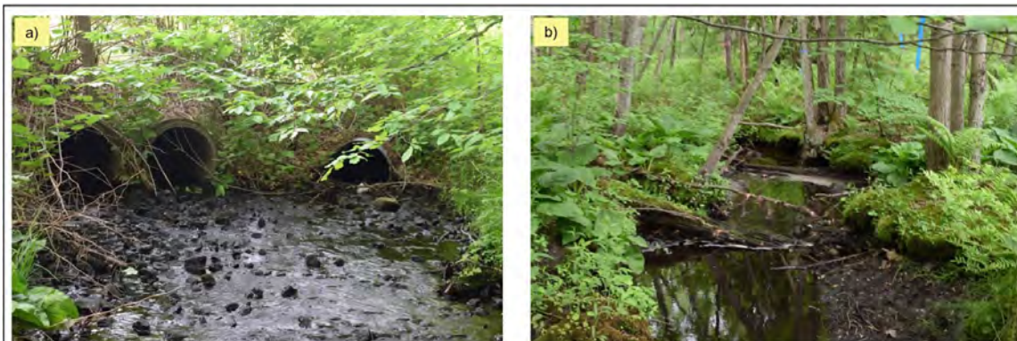
Figure 6. Reach 6 has a) an artificially armored bed at the outlet of the Baribeau Dr. culverts but b) further downstream appears in a near natural state.
