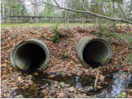
cul03 Inlet Pipe
