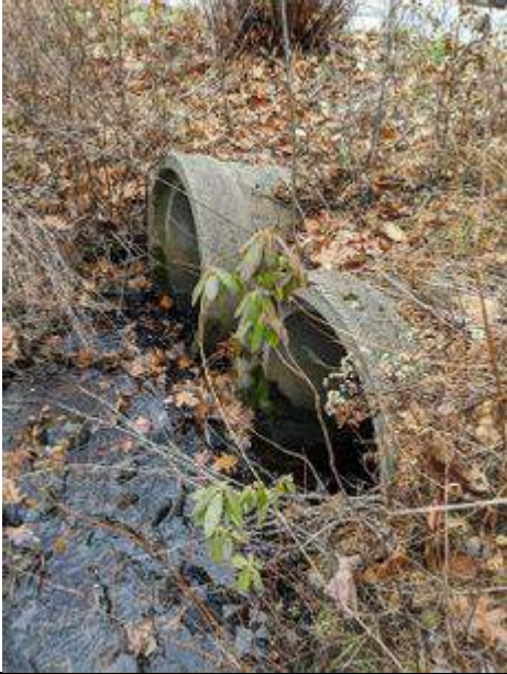
cul05 Inlet Pipe
