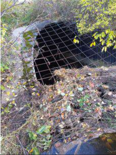
cul29 Inlet Pipe
