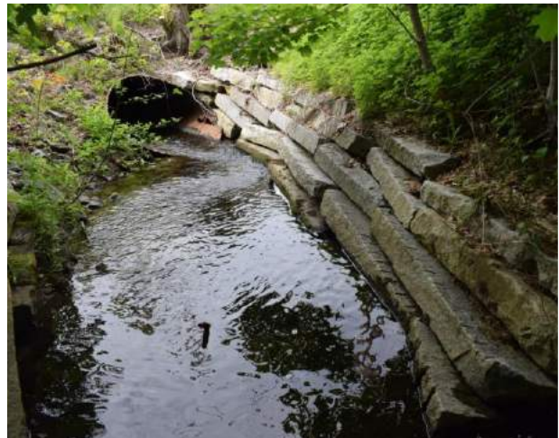
Upstream view of granite blocks and Maine Street culvert outlet of Reach 9 during the geomorphic survey. Photo: John Fields
