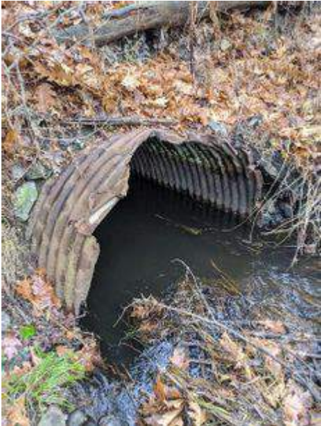
cul23 Inlet Pipe
