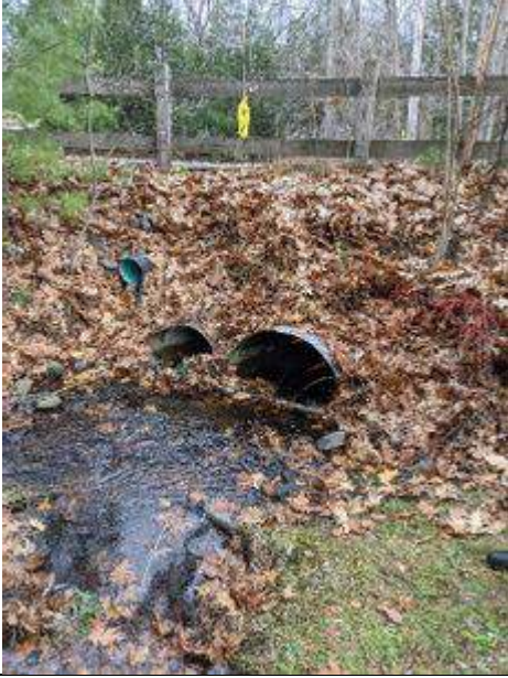
cul10 Inlet Pipe
